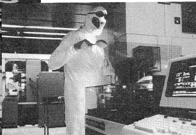
State-of-the-art wafer fab clean room facilities at Harris are maintained up to a class 10 level.
